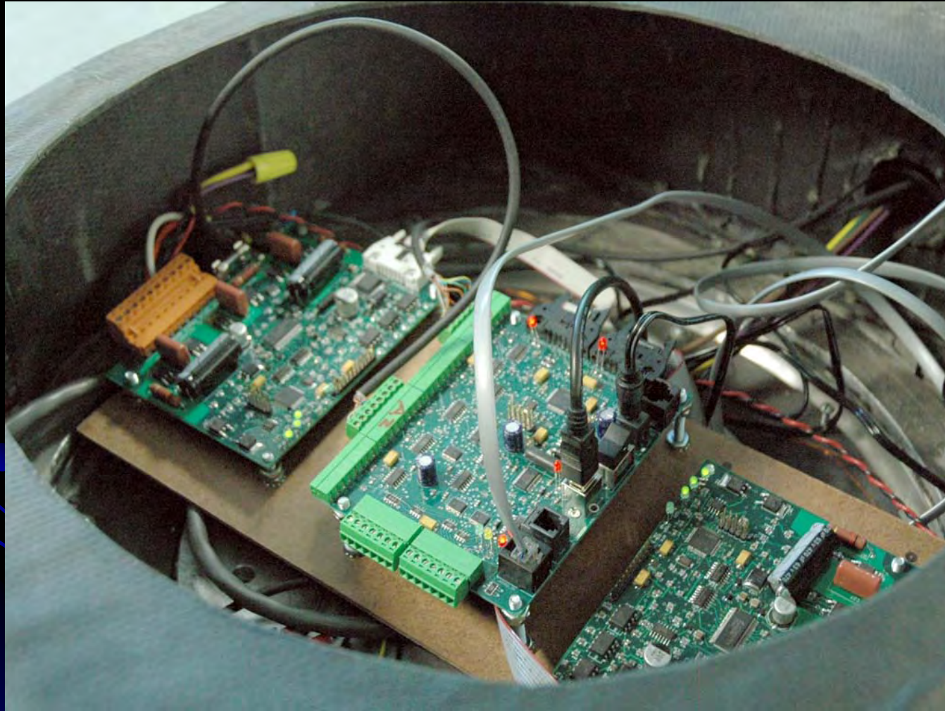
SciTech circuit boards in base of Cal Poly 18 fork assembly
